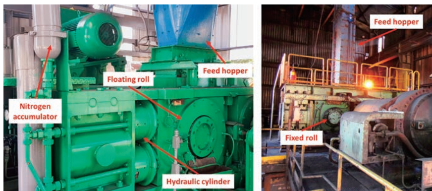
Fig. 1 Pilot-scale HPGR (left) and industrial-scale HPGR (right) used in the experimental campaigns.
