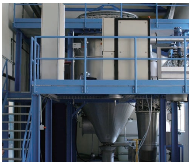
Fig. 6 Front view of the FSP pilot plant during installation at ARCI (Hyderabad, India) for production of several kg/h of nanoparticles with the baghouse filter for nanoparticle collection ( \sim 50 \text{ m}^2 filtration area) at the back in the center, the stirred tank for precursor preparation on the right and the control cabinet for process automation on the left side of the platform.
